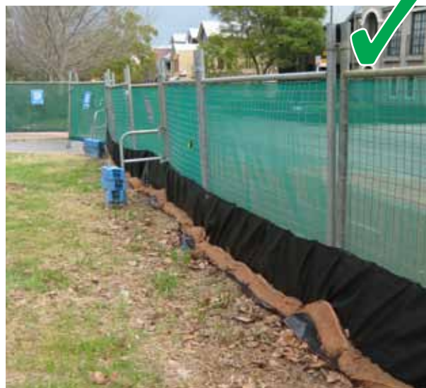
Secure the geotextile material to the perimeter fence to a minimum height of 600 mm.
