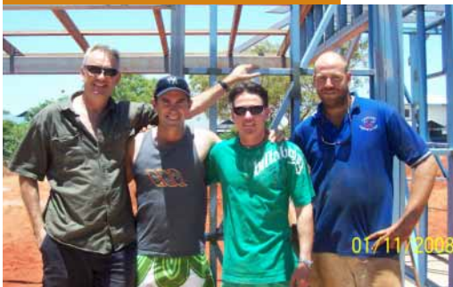
The Foundation's Patron, Justin Langer inspecting the progress in November and the house prior to Christmas. R-L Darryn Wardle, Justin Langer, Troy Dahlstrom and Steve Norman
